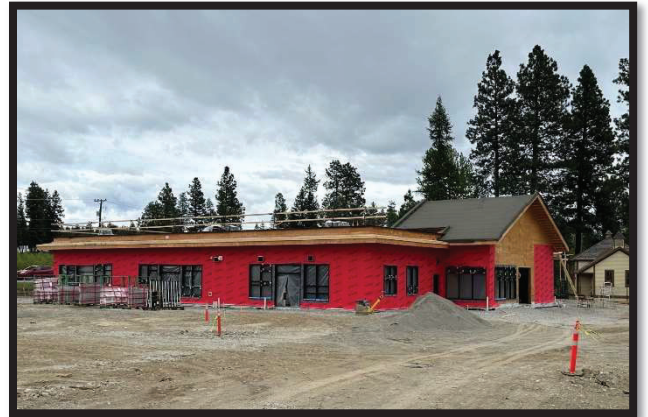
Under construction – The Marysville Child Care Facility is expected to be completed this fall.
